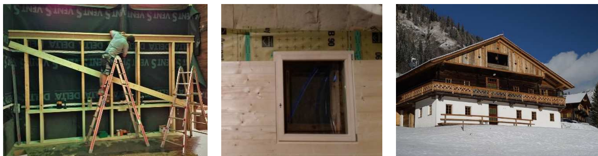
Figure 8: left: Black wind paper and the frame construction for the OSB panels in "Hof Neuhäusl" © DI Hans Peter Gruber; right: New block wall on the inside of the "Giatlashaus". The space between the old log wall and new log wall was insulated with sheep wool. ©Benjamin Schaller
