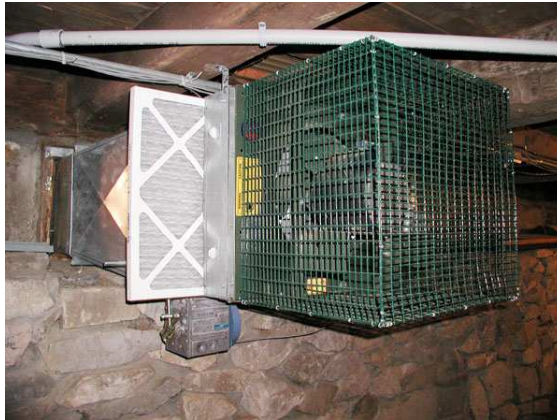
Figure 7. Basement intake fan assembly showing dust filter pulled out.
