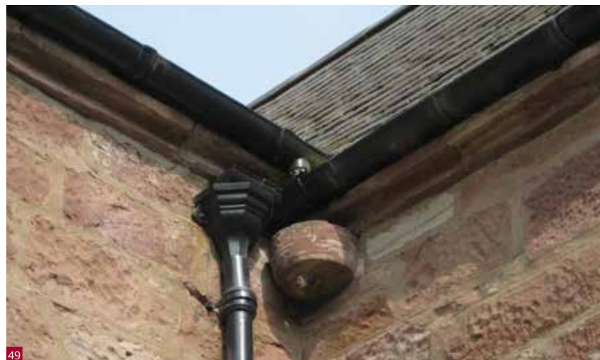
Fig. 49 Works to this building have neglected to reuse the original stone rainwater bracket, resulting in an overly complex arrangement.
