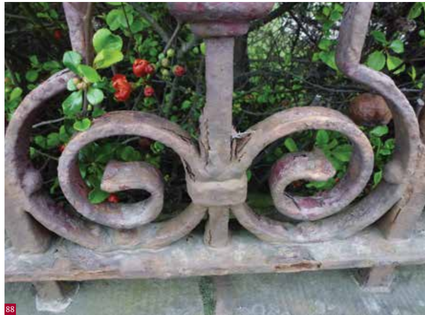
Fig. 88 Example of poor repair and corrosion of iron railings.
