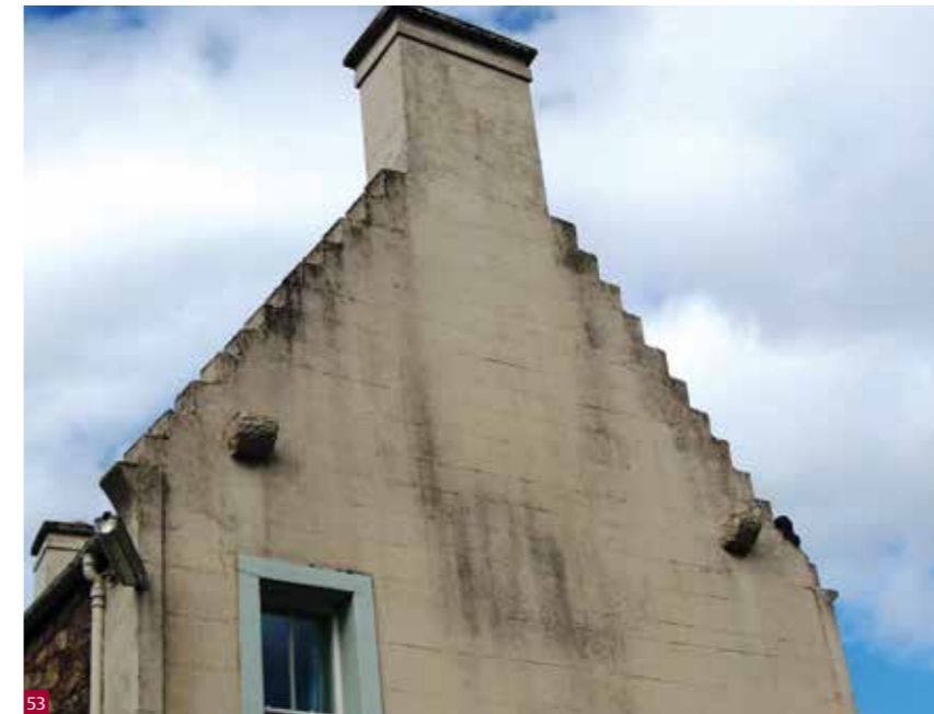
Fig. 53 A lack of protective water shedding detailing has led to staining, and progressive crazing of this cement-rendered gable.
