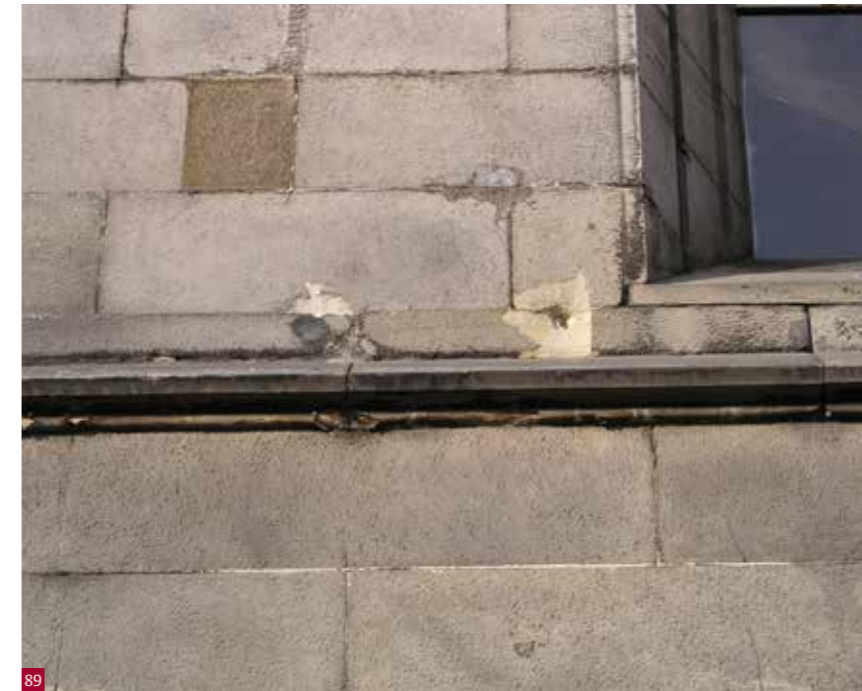
Fig. 89 Open joints in masonry have allowed water to penetrate, leading to corrosion of embedded iron cramps and fracturing of stone.
