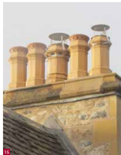
Fig. 15 A poorly maintained chimney stack.
