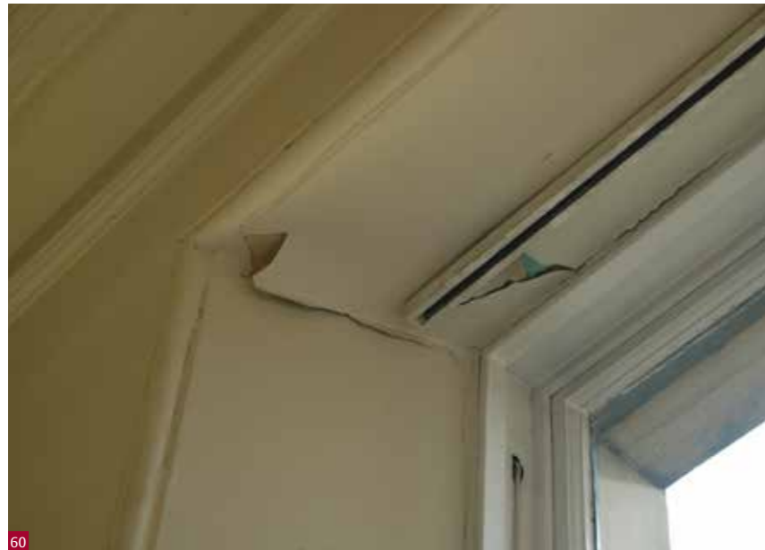
Fig. 60 Internal decorative damage, caused by water ingress.
