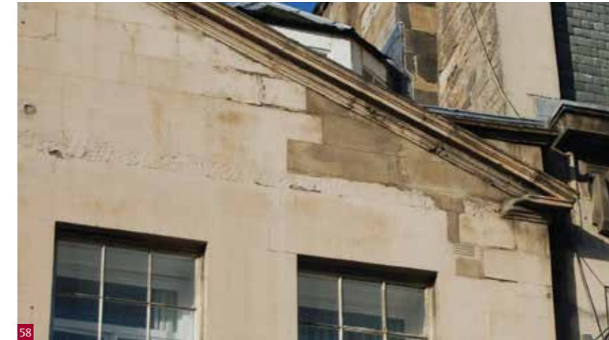
Fig. 58 A traditional masonry elevation where the cornice has been removed.
