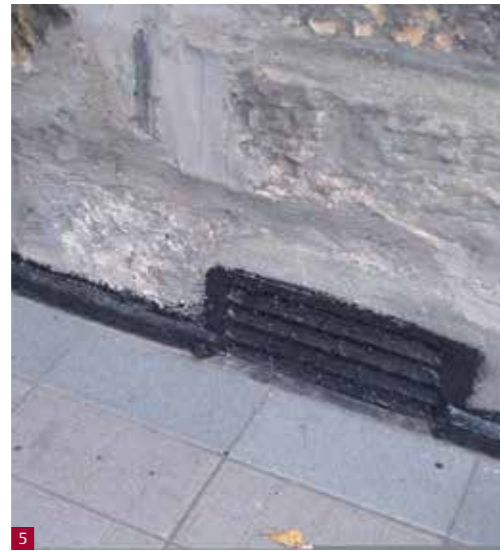
Fig. 4 Water ingress has led to progressive failure of the chimney and masonry below.
