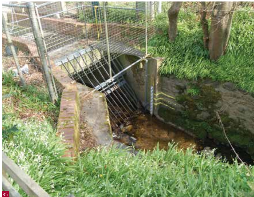
Fig. 85 An urban drainage feature vulnerable to blockage and flooding.
