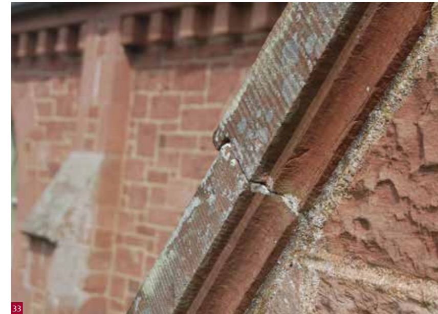
Fig. 33 Raised moulding on upper skew copes to ensure effective water run-off and prevent water ingress.
