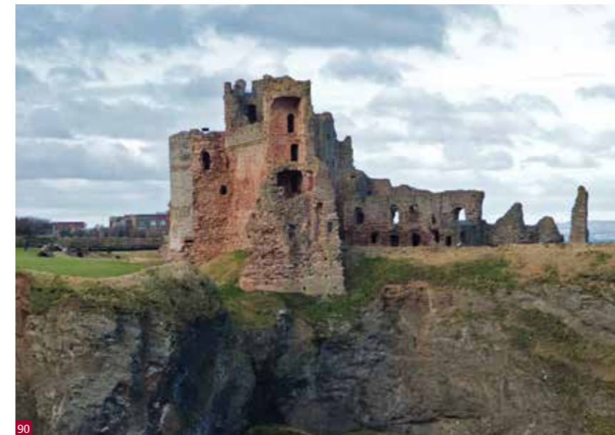
Fig. 90 Coastal erosion at Tantallon Castle, North Berwick.
