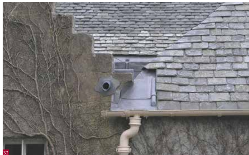
Fig. 32 Enhanced lead detailing, such as the use of a storm roll, can be conspicuous, but is an effective way to improve rainwater disposal in areas of high water flow.
