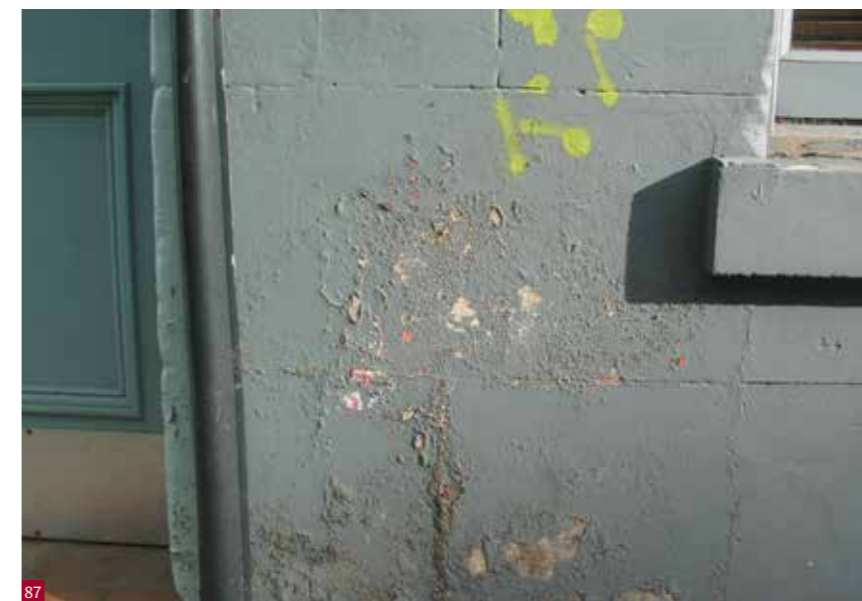
Fig. 87 Blistering external paint due to trapped moisture behind.
