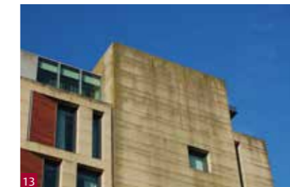
Fig. 13 Poor detailing on a modern building in Edinburgh has led to staining of the masonry.
